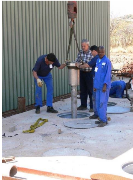
Figure 3: A new SAFARI-1 storage vessel being lowered into a borehole during the 2006/7 extension
