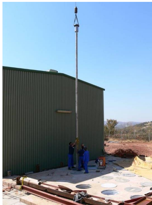
Figure 2: Placement of a new SAFARI-1 storage vessel into a borehole during 2006/7 extension
