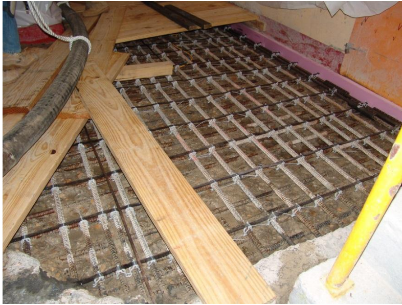
Figure 5-5. Titanium Ribbon Mesh Anode installed in Concrete Repair using Plastic Rebar Clips
