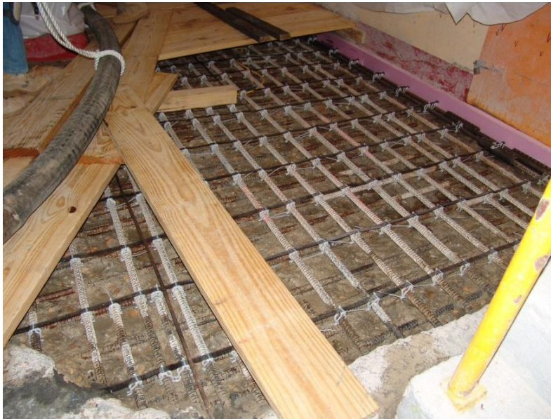
Figure 8: Titanium Ribbon Mesh Anode installed in Concrete Repair using Plastic Rebar Clips (Source: Corpro Companies, Inc.)
