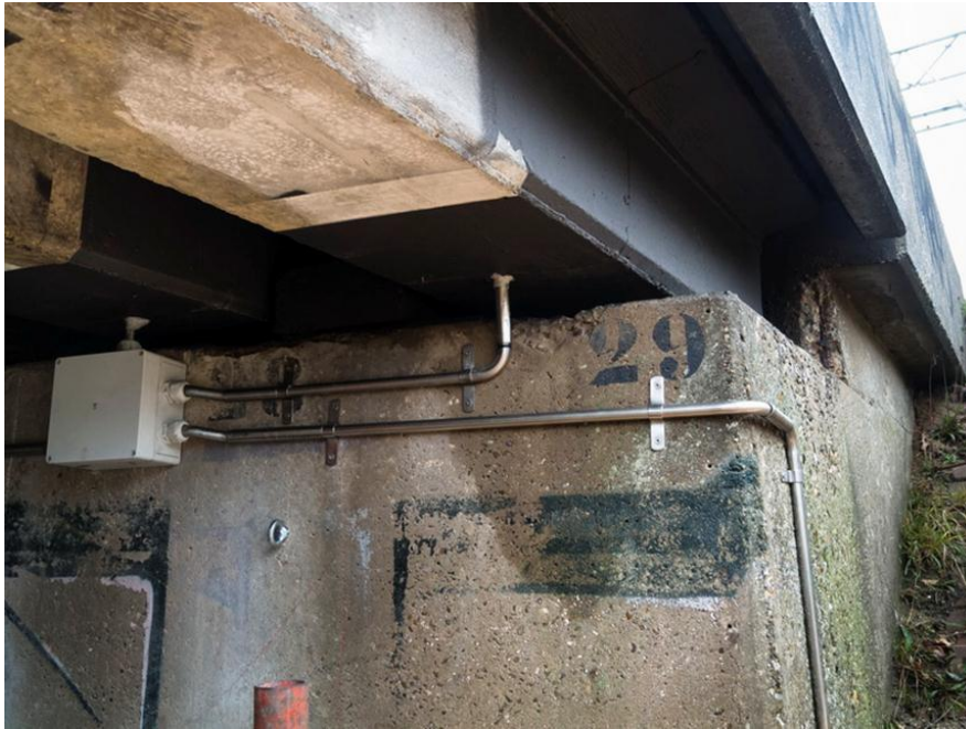
Figure 6: Conductive coating (black) CP applied to ends of post-tensioned bridge deck beams and stainless steel conduits to power supply box
