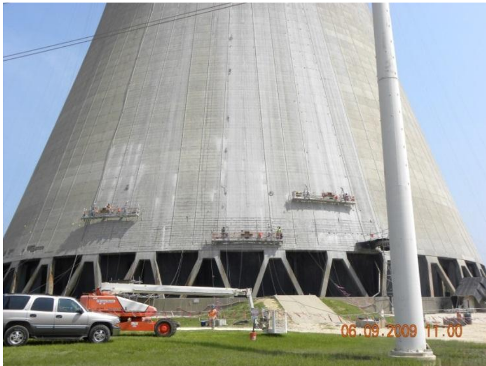
Figure 10: Installation of an Impressed Current System on a Hyperbolic Cooling Tower ( [REDACTED] )
