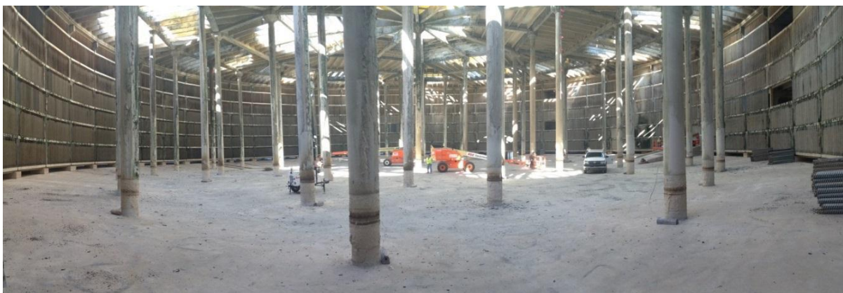
Figure 5-1. Galvanic Anodes at Base of Cooling Tower Columns
