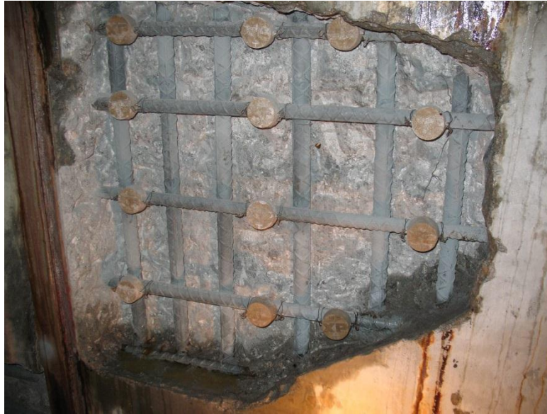
Figure 5-4. Point Type Zinc Anodes installed in Concrete Repair of Seawater Intake Structure
