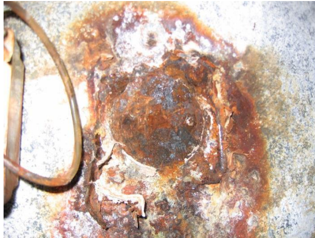
Figure 5-3. Thermally Sprayed Zinc Anode Connection Failure in Seawater Intake Structure
