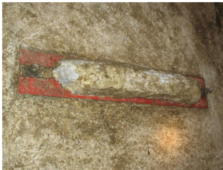
Figure 5-2. Galvanic Anode in Circwater Cooling Tunnel
