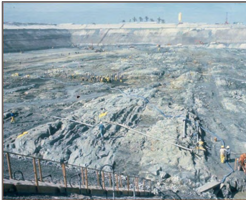
Figure 9-93. Photo of excavation to top of rock at the Koeberg NPP (Eskom, 1977)
